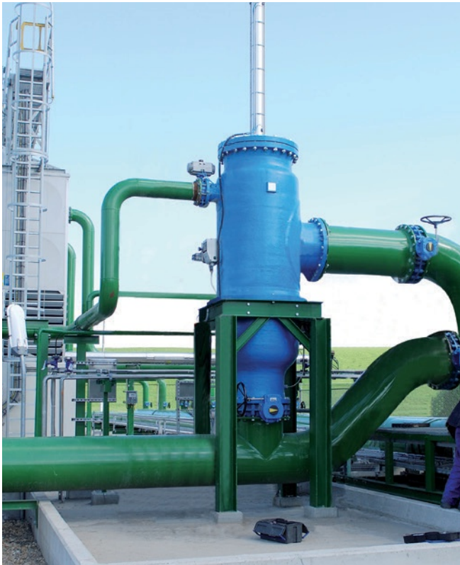
24"/DN 600 KAF® Filter – Bioethanol plant
