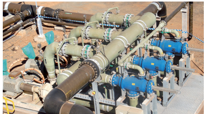
3 x 16"/DN 400 KAF® Filter – desalination
